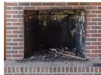
Thermal boiler and fireplace insulations
