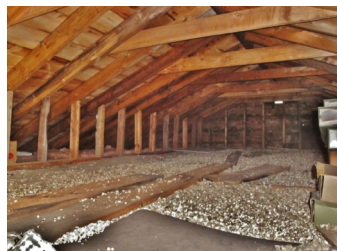
Vermiculite insulation, ceiling tiles and coatings
